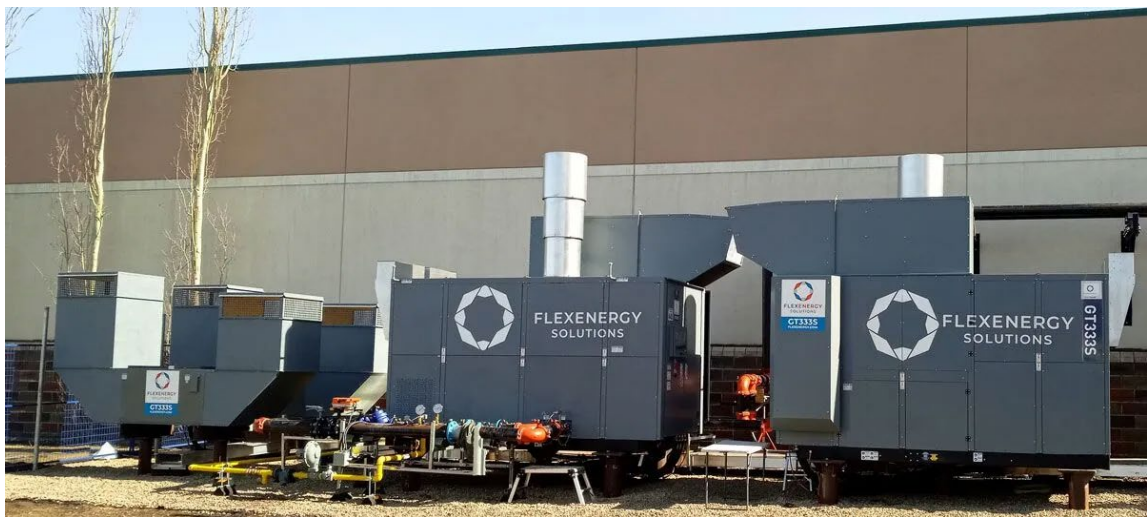
Figure 1 - Flex Energy's turbines running the power for Grand Prairie EastLink Centre 3
