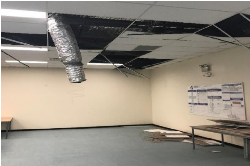
Photo 1: Ridge Camp damage
