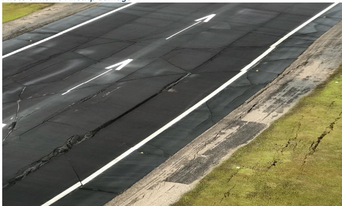
Photo 3: Komo Airstrip damage
